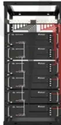
Cabinet and rack installation display
