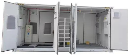
1075KW HH ESS
