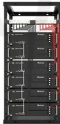
Cabinet and rack installation display
